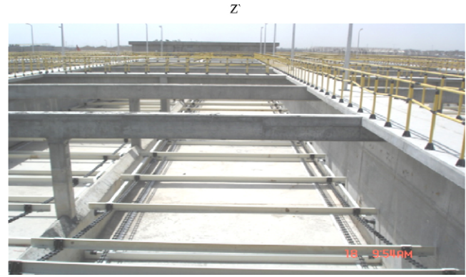
Fig. 1. Longitudinal sedimentation basin in the water treatment plant.
